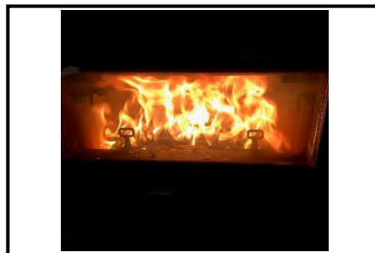
Typical High Fire Coal Bed
